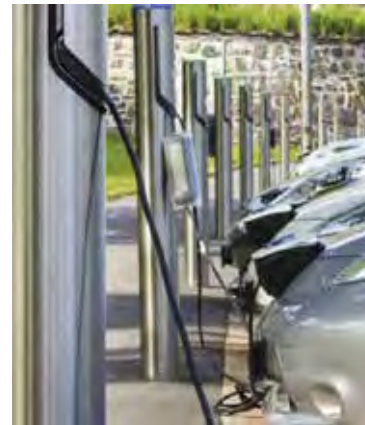
Electric car charging points
