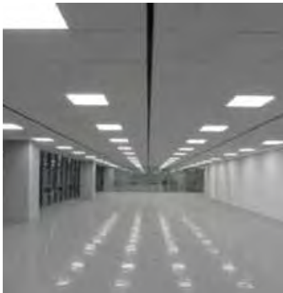
Highly efficient LED lighting
