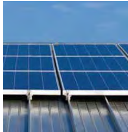
Roof mounted photovoltaic (PV) arrays
